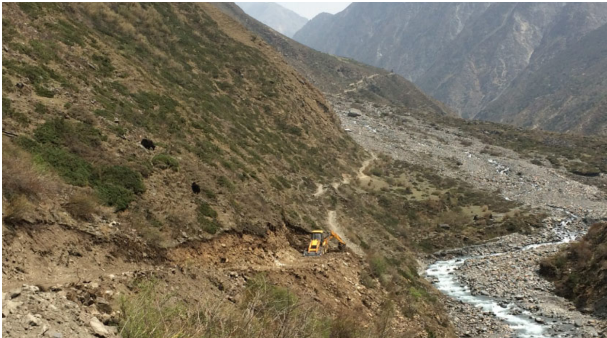
Photo 1. A bulldozer haphazardly digs a road out of a hillside in Nepal's Tsum Valley. Eventually this road will reach all the way to Tibet. Photo: Chris Czarnecki
