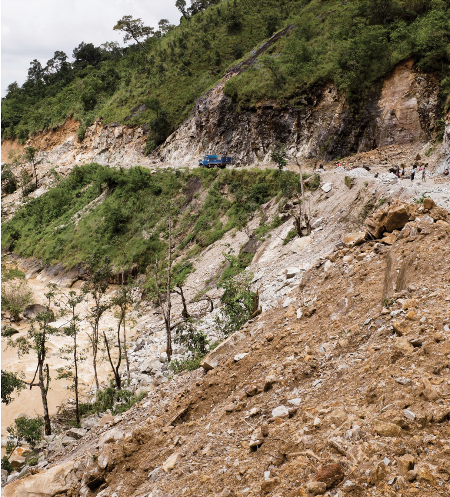
Soil erosion and minor landslides can be observed along the road.
